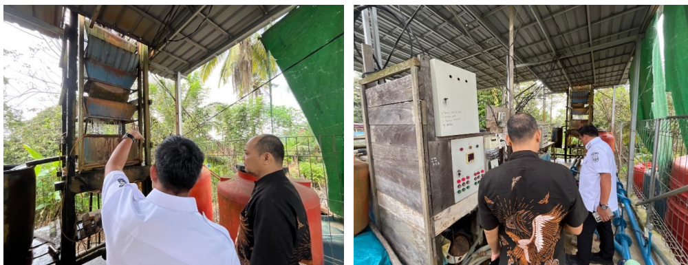
Figure 1. Initial infrastructure of the Water Treatment Plant (WTP) in the development of a clean water supply system in Batuah Village
